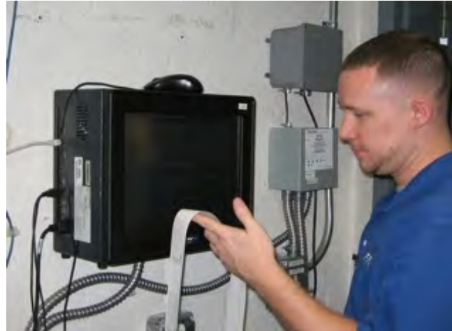
FFM began looking for a better fuel management system for improved monitoring and leak detection capabilities.
